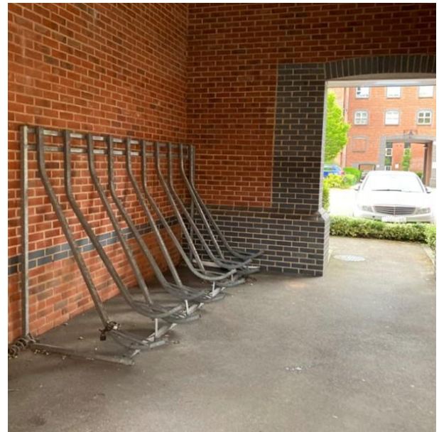
Cycle parking racks for long-term parking at residential flats. Whilst the area is covered, there is no natural surveillance of the area, and no way for residents to double lock their bikes, leaving them vulnerable to theft. The style of stand requires a certain amount of upper body strength, therefore making this style not suitable for all to use.
